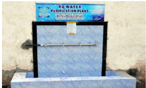
RO water purification plant installed under IAEA project RC-24975 on Nov. 22, 2023
